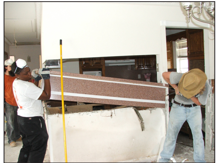
My'eka and Austin pry a counter top loose from a home in the town of Jean Lafitte, which is south of New Orleans. The group gutted a total of five houses in four days of work; all the houses had been flooded by Hurricane Ike this year.
