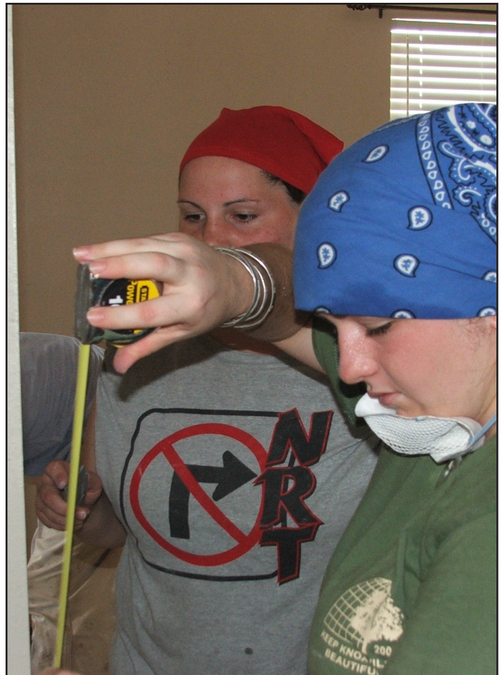
Megan Shapiro, assistant to Dr. Irene Hodgson and fellow New Orleans traveler, measures the wall as Tara stands by ready to mark it for the chalk line used to cut out the bottom half of the sheet rock so the house can dry out and be redone.
